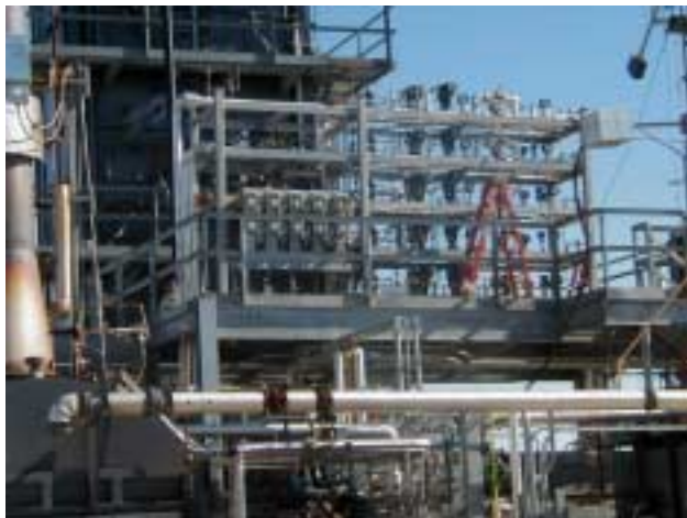
Figure 1 - Test Furnace Metering Skid
